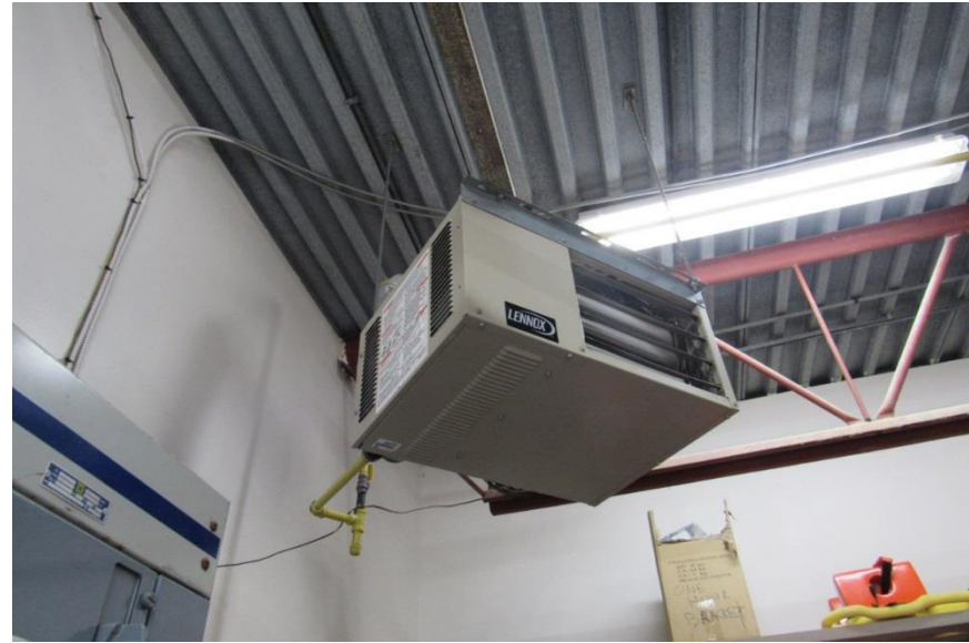
Photo #M8: Gas-fired unit heater at the Pool.
