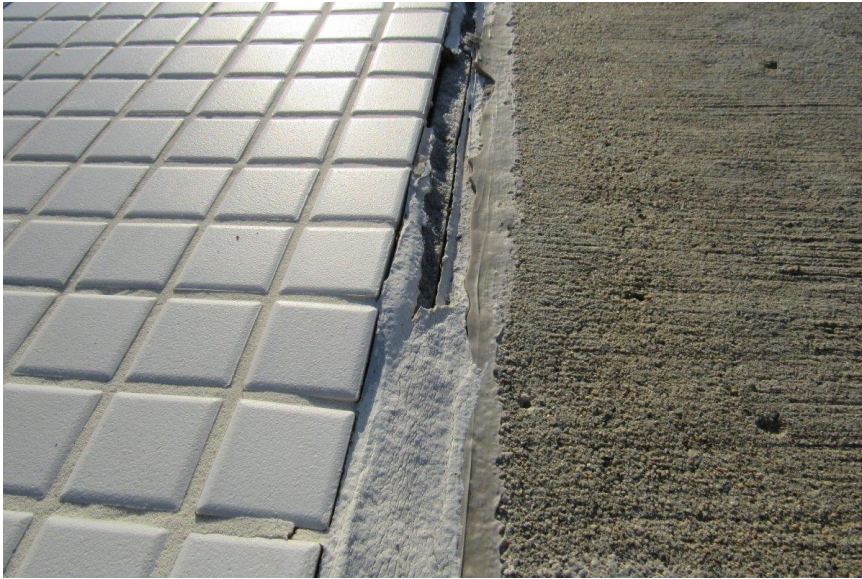
Photo #S7: Cracks at Pool Deck.
