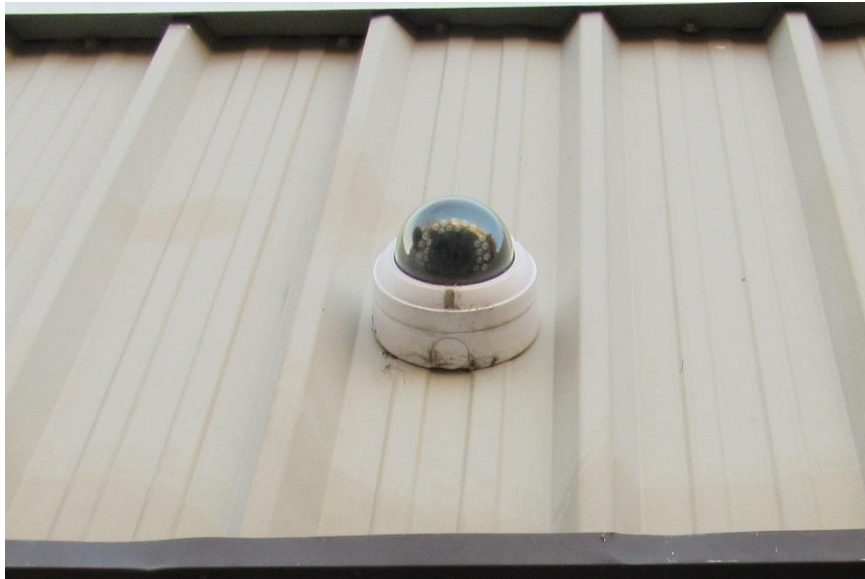
Photo #E9: Surveillance camera at the Pool.
