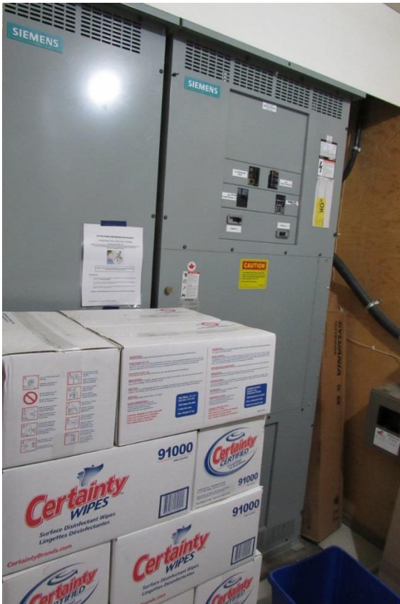
Photo #E1: Primary electrical panelboard at the Community Centre.
