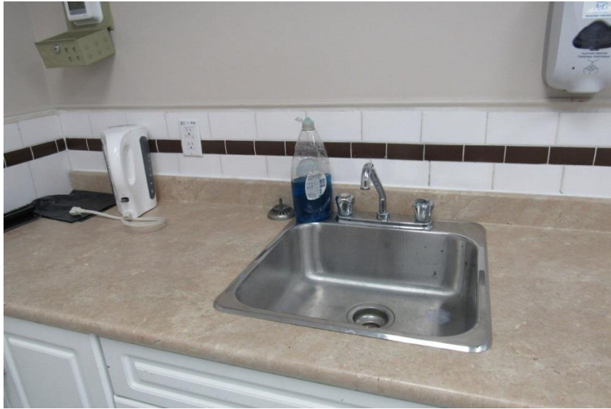
Photo #M5: Counter-mounted stainless-steel sink.
