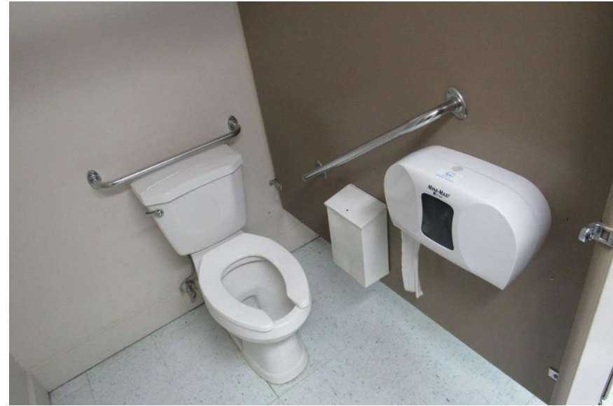
Photo #M4: Typical vitreous china flush tank toilet.
