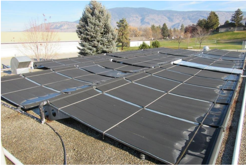
Photo #M3: Solar collectors on the roof of the Pool building.
