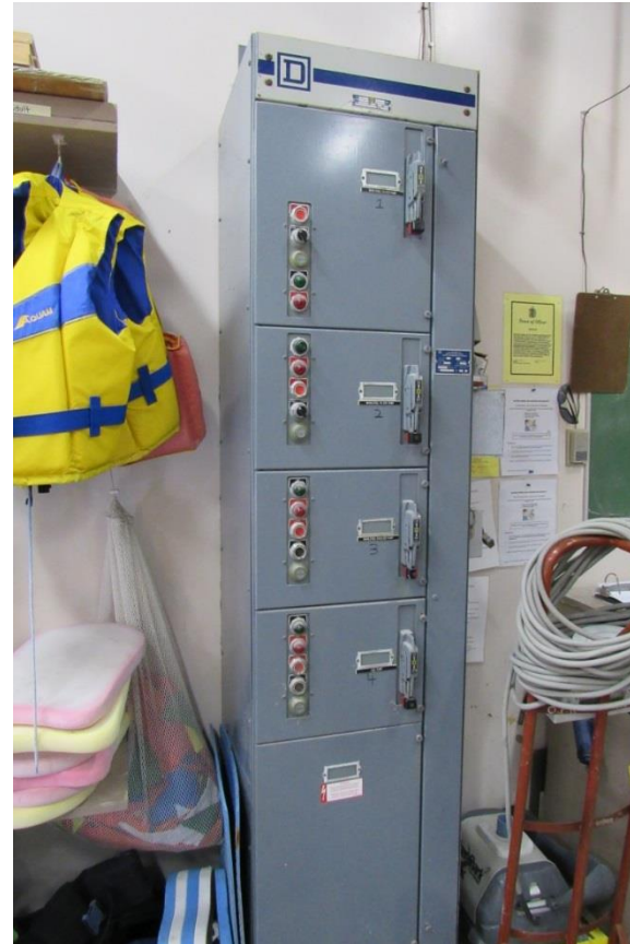
Photo #E4: Motor control centre at the Pool.
