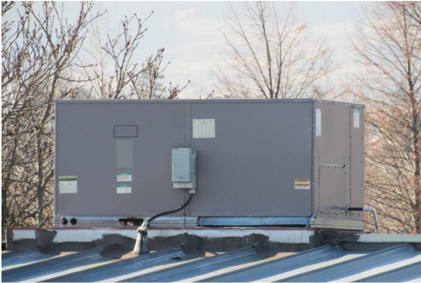
Photo #M7: Gas-fired RTU at the Community Centre.
