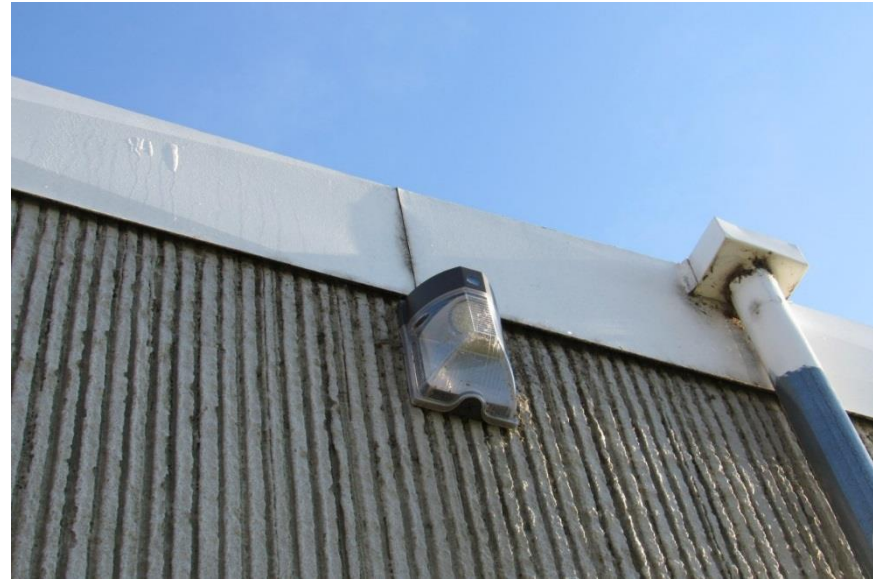
Photo #E6: Exterior LED lighting fixture at the Pool.
