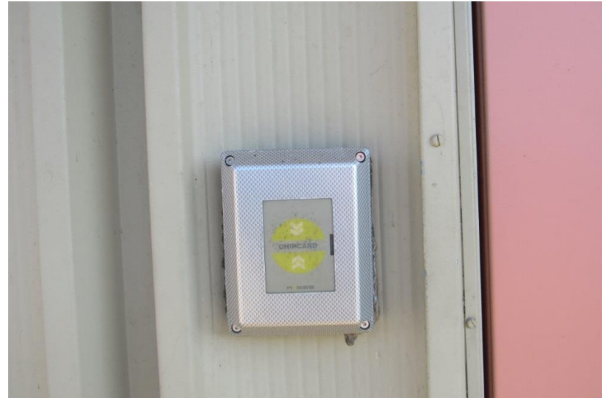
Photo #E10: Proximity card reader at the Community Centre.
