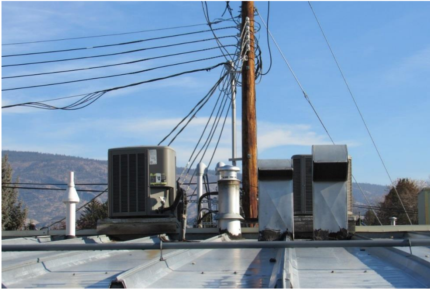
Photo #M11: Condenser units at the Community Centre.
