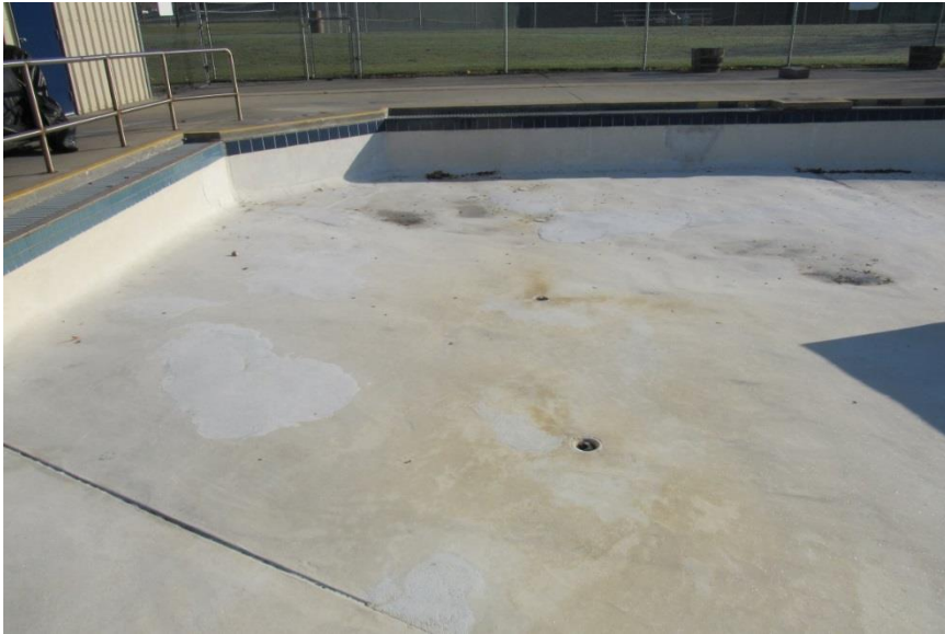
Photo #A3: Patched Pool basin.
