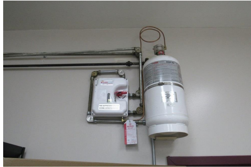
Photo #M12: Kitchen fire suppression system.
