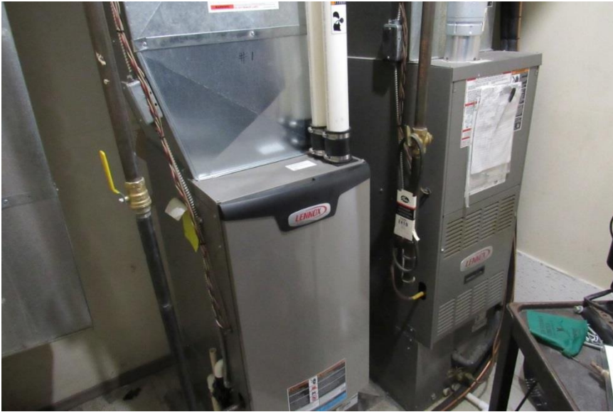
Photo #M9: Gas-fire furnaces at the Community Centre.
