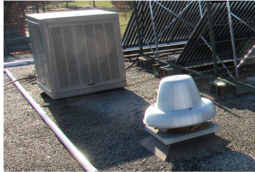
Photo #M10: Evaporative cooler and exhaust fan at the Pool.
