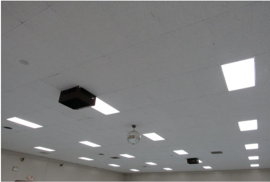
Photo #E5: Interior fluorescent lighting at the Community Centre.
