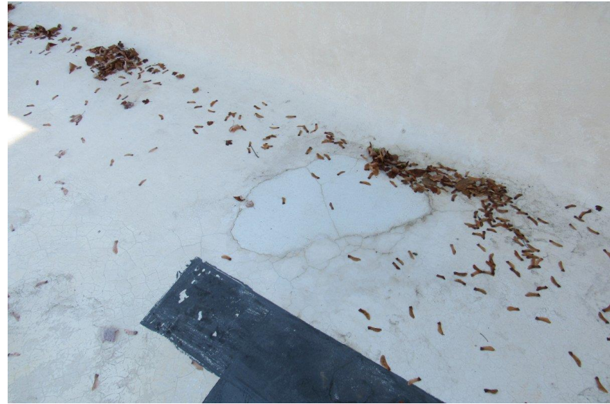
Photo #S8: Cracked Pool Basin.
