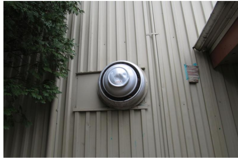
Photo #M8: Wall mounted fan.
