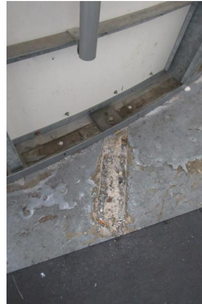
Photo #S2: Spalling concrete just outside the rink.
