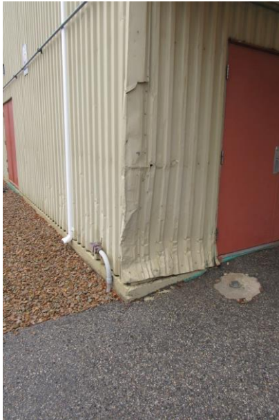
Photo #A5: Metal siding damages at the south-east corner of the building.
