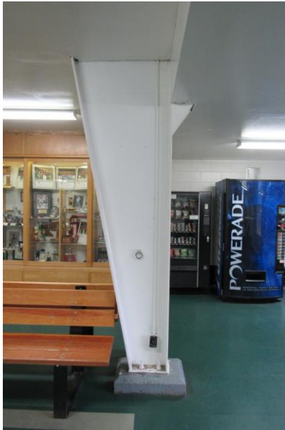
Photo #S3: Typical interior structural steel column.
