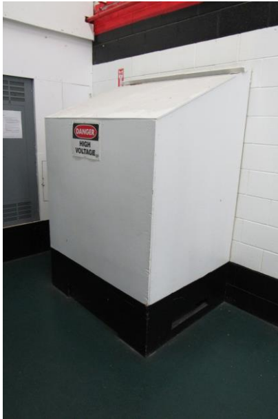
Photo #E1: Encased interior transformer.
