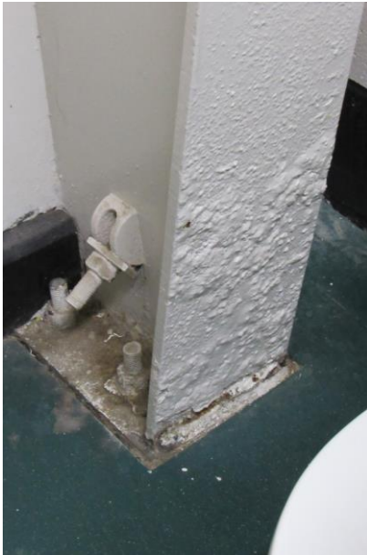
Photo #S5: Rusting observed in one of the change rooms.
