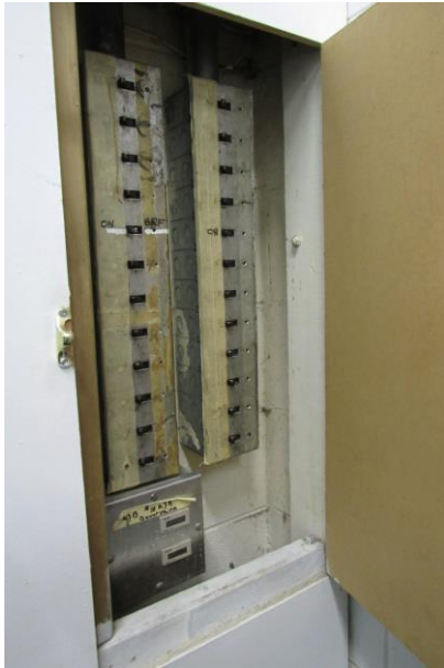
Photo #E3: Original, electrical sub panel.
