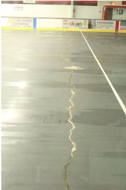
Photo #S1: Cracked SOG ice rink floor.
