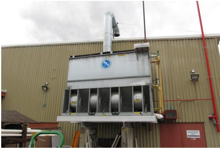
Photo #M7: Condenser for the ice plant.
