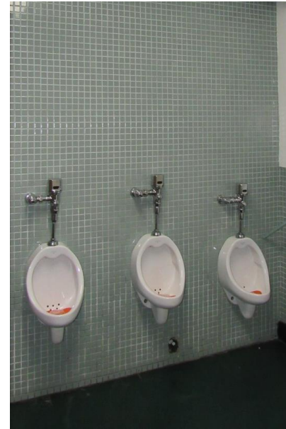
Photo #M2: Typical plumbing fixtures.
