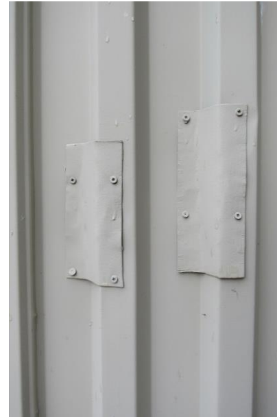
Photo #A6: Typical metal patches observed on metal siding.
