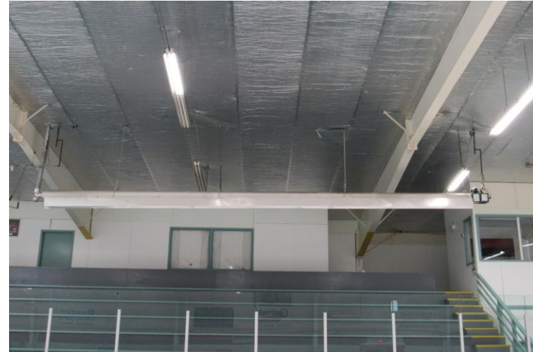
Photo #A18: Ice arena spectator benches and exposed roof insulation.
