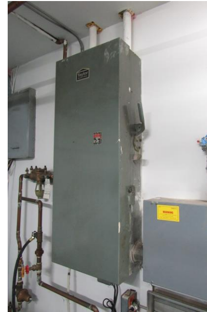
Photo #E2: Main switch located in compressor room.
