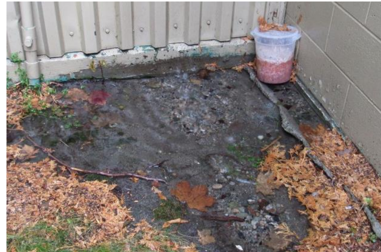
Photo #A12: Water pooling near the main entrance caused by leaking roof gutters or downspout.
