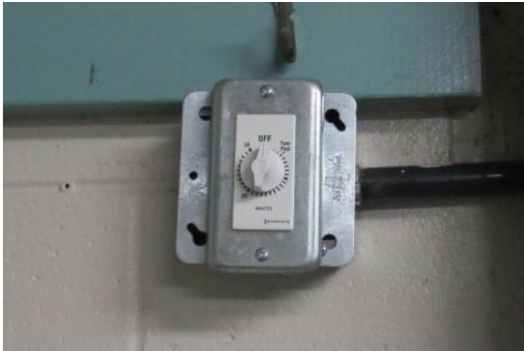
Photo #M5: Timer used to control the unit heaters in the dressing room.
