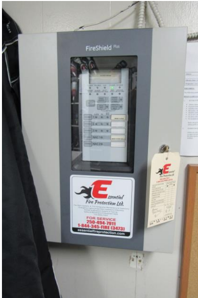
Photo #E9: The fire alarm panel.
