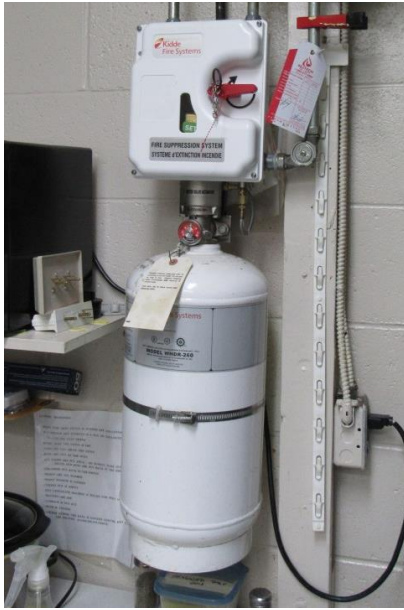
Photo #M9: Chemical fire suppression system.
