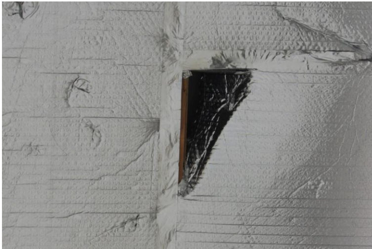
Photo #A19: Typical minor damage on arena ceiling (batt insulation).
