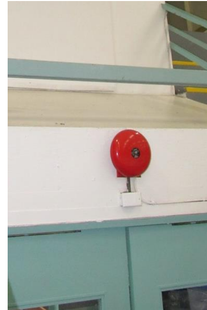
Photo #E10: Fire alarm bell.
